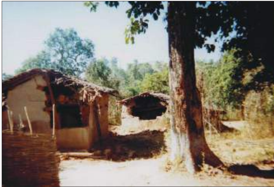
A house damaged by wild elephants in Chhattisgarh
