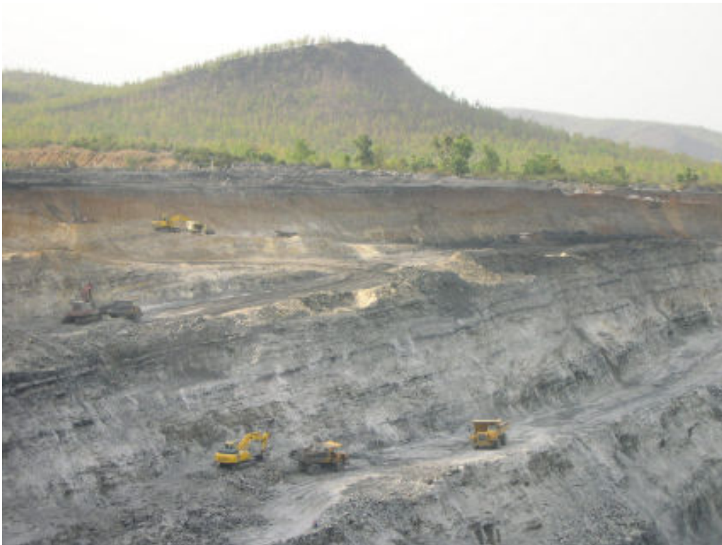
Mining activities going on at the Damodar Valley wildlife habitat near Hazaribagh NP
